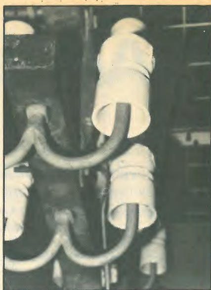
Fig. 9. Simple and effective conical skirts of common British telegraph pole insulators, in use for nearly a century, and only now recently adopted for marine use, Figs. 10 and 11.
